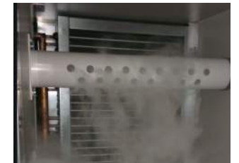
Humidification (Steam entering the air stream)
